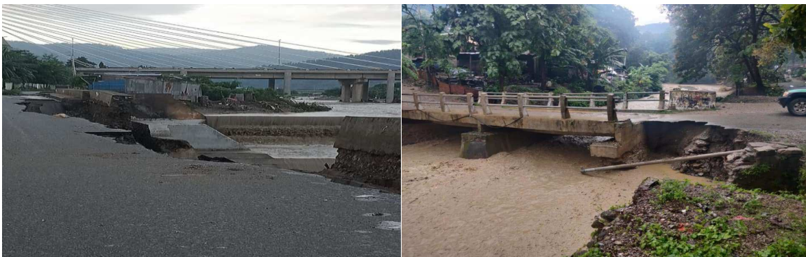
Figure 3. Damage to public infrastructure, 4 April 2021
