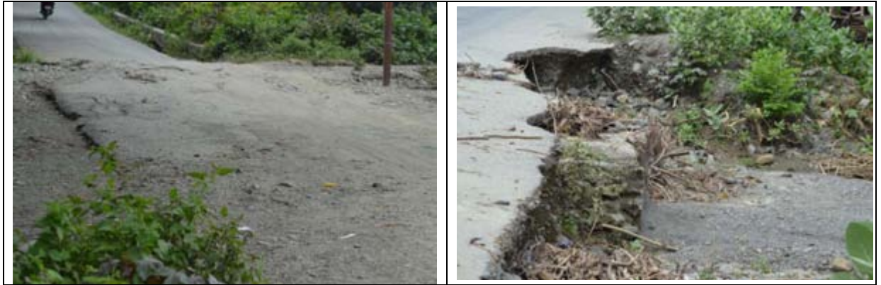
Plate 2 Left photo shows sediment deposited on the road pavement by surface runoff overtopping the road pavement and right photo shows deep undercutting along the cross drainage structure and erosion of road pavement
