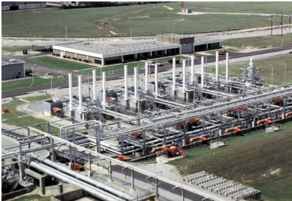
Figure 26. Seven Submerged Combustion Vaporizers, Lake Charles, La., Terminal
