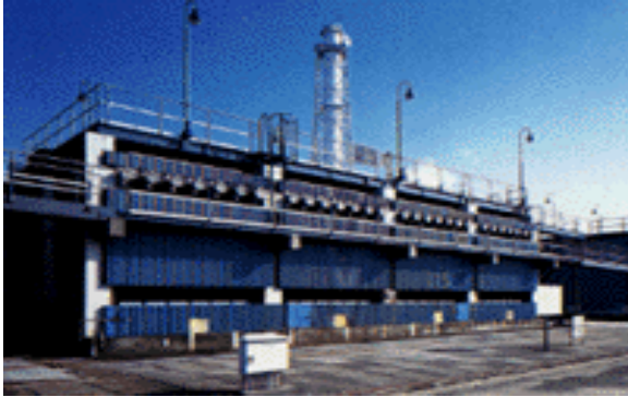
Figure 25. Open Rack Vaporizer
