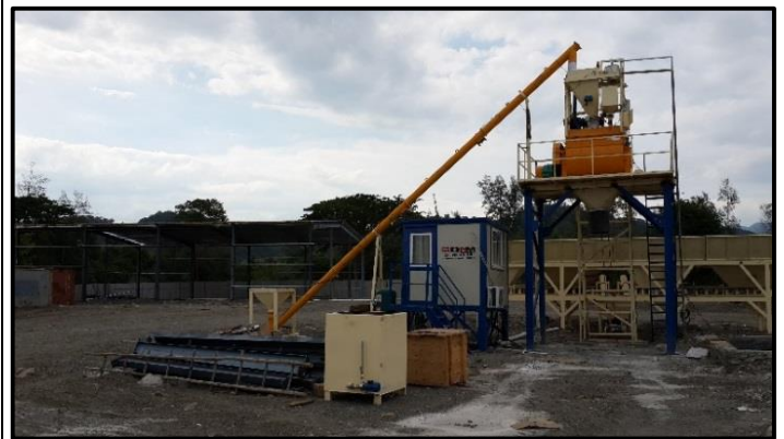
Branch 1 Concrete Mixing Plant
