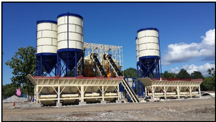
Branch 2 Concrete Mixing Plant
