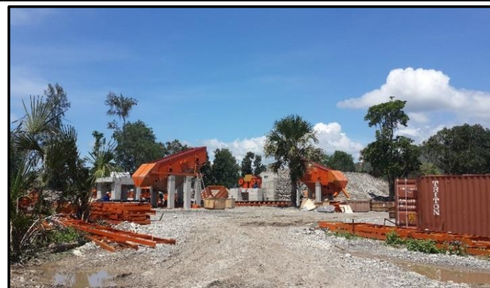
Stone Crusher Screen & Washer in Branch 2
