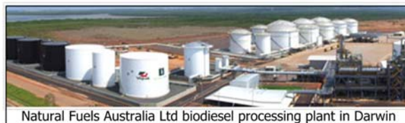
Natural Fuels Australia Ltd biodiesel processing plant in Darwin
